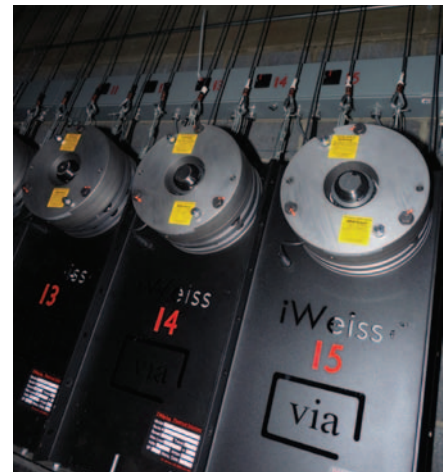
iWeiss Via Winches installed at Riverside Church's South Hall
