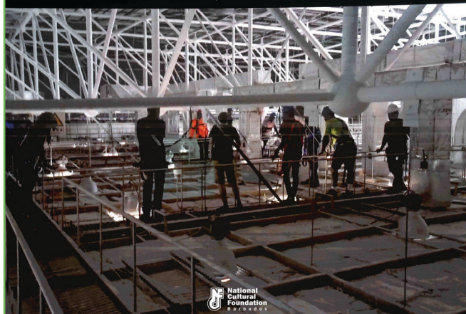
Image description: Workers in safety gear stand on a platform beneath a network of steel trusses, highlighting teamwork and engineering precision in a large architectural space.
