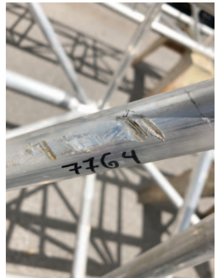
Figure 2 – Damage to truss diagonal caused by a forklift while truss was being unloaded from a truck. It isn’t uncommon to see diagonals broken out of the module due to operator error.
