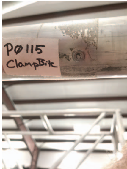
Figure 1 – Typical damage caused on a truss chord from the use of a standard lighting clamp without any protection installed on truss. Most manufacturers recommend against using lighting clamps on truss, or only using when a protector is placed on truss.
