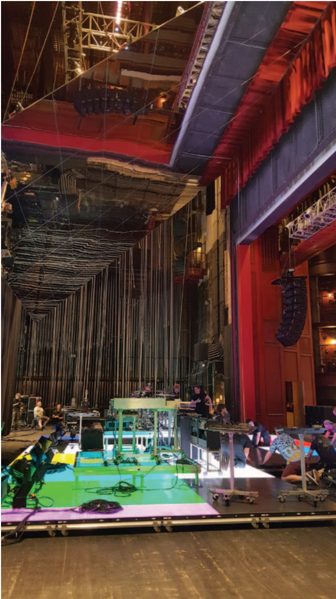
Mother grid rigging for 2.8T slanted mirror provided by PRG at the Fillmore Miami Beach for the band Phoenix's 2017 tour.
