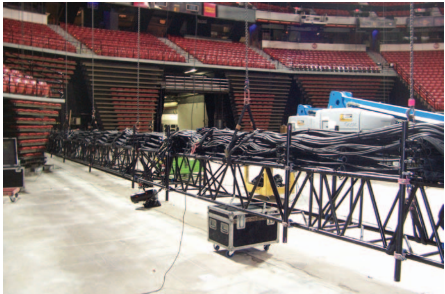
One NBA All-Star Game used 150'+ runs of 70+ multi-cables requiring air-space for heat dissipation. To accomplish this, Rob Baxter made 2" PVC "roller-bearings" to support, space, and slide the nearly three tons of cable. They called this the "Vegas Cable Condo."
