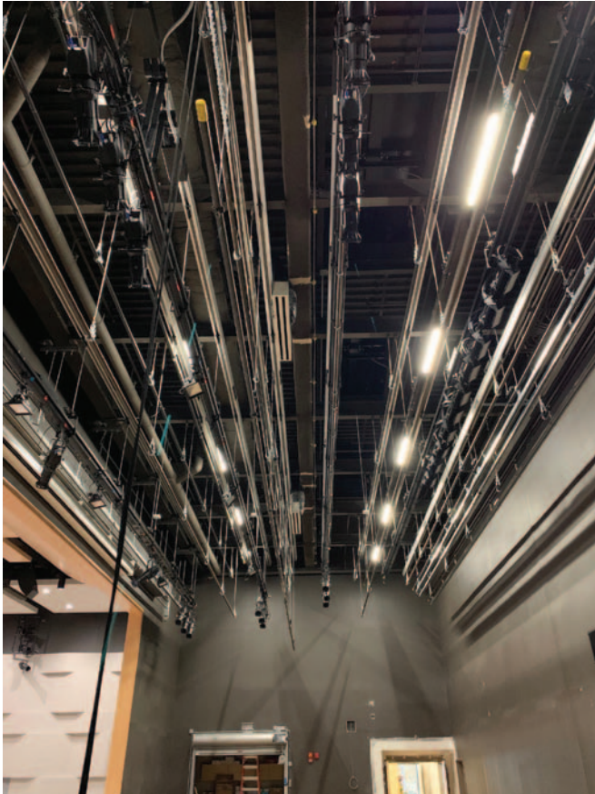
Barbizon installed the rigging system in the East Providence High School Performing Arts Center in Rhode Island. It was completed in November 2021.
