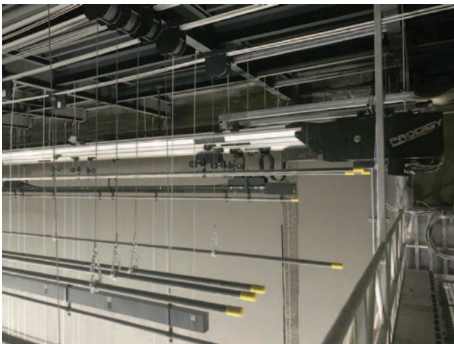
Durfee High School in Fall River, MA, uses a hybrid rigging system of counterweight and motorized line sets. It was completed in December 2021.
